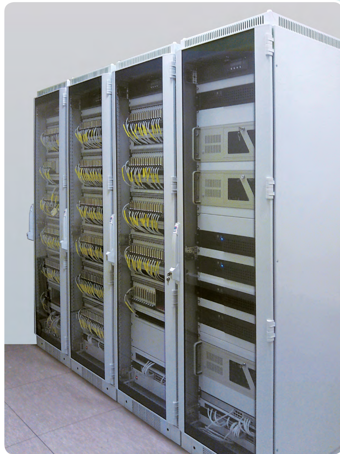
Racks of measurement system
