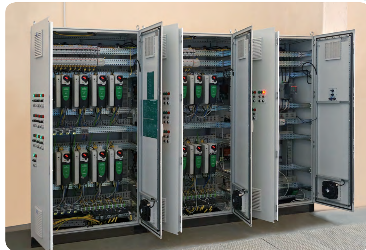
Power control cabinets
